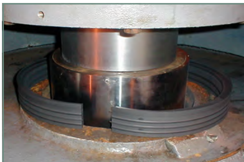
SpiralTrac installation in a large influent pump at a wastewater treatment plant
