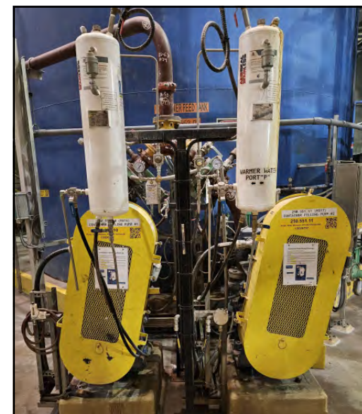
Original Double Seal Setup with Barrier Fluid Tanks
