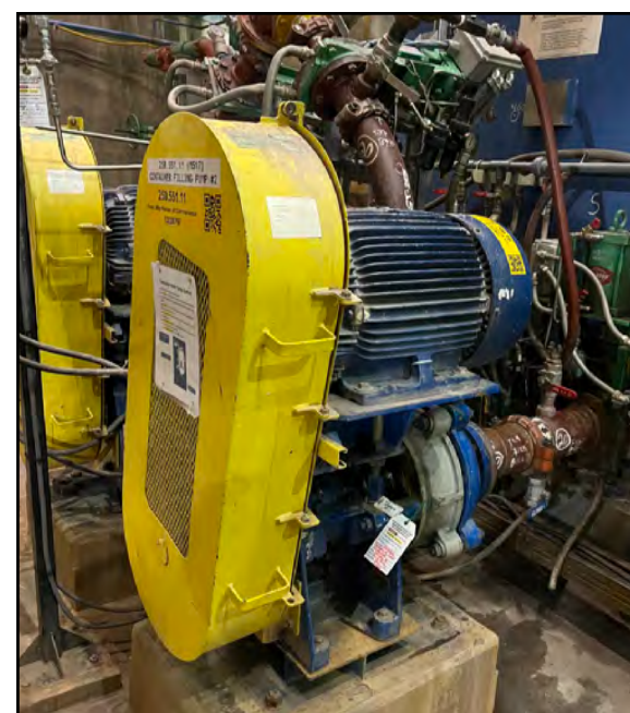
No Flush Chesterton Solution Installed
