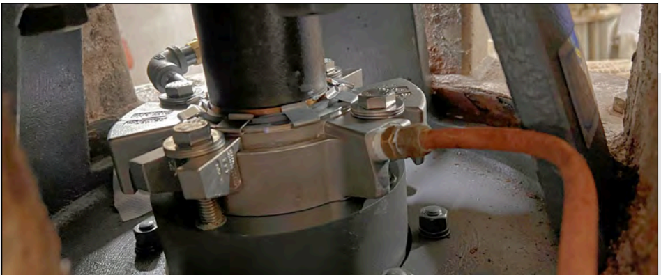
Chesterton solution Installed and running great without issues
