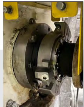
Chesterton Solution installed
