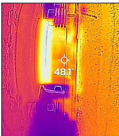
Thermo camera showing heat measurements during operation
