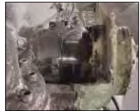
Chesterton Solution installed
