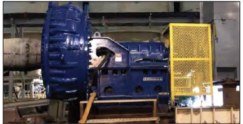
Large Pump required adjustment every few days due to severe leakage
