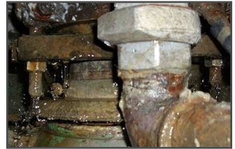
Leakage problems with original sealing setup
