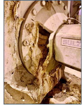
Excessive product leakage with original hydrodynamic seal
