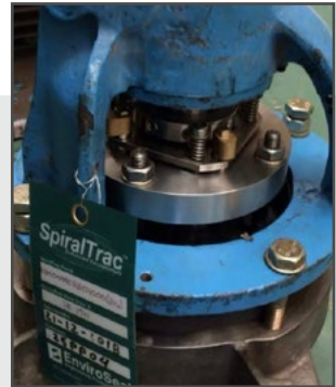
Assembled Rheinhalte pump showing 170 seal and SpiralTrac green tag
