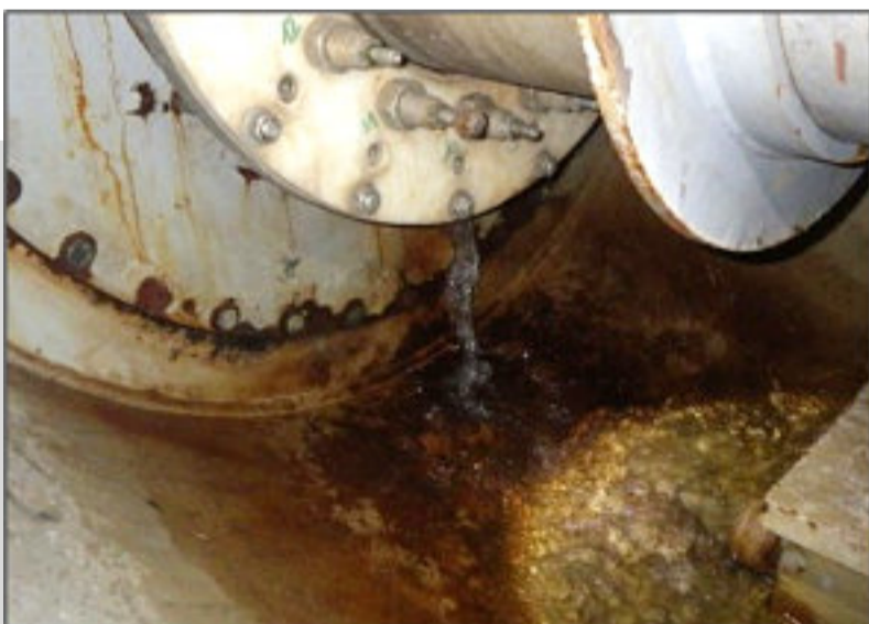
Excessive leakage with original segmented seal
