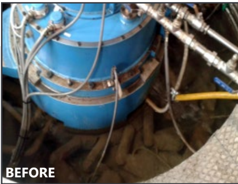
Turbine seal failure with OEM solution
