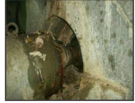
Excessive product leakage at the gland
