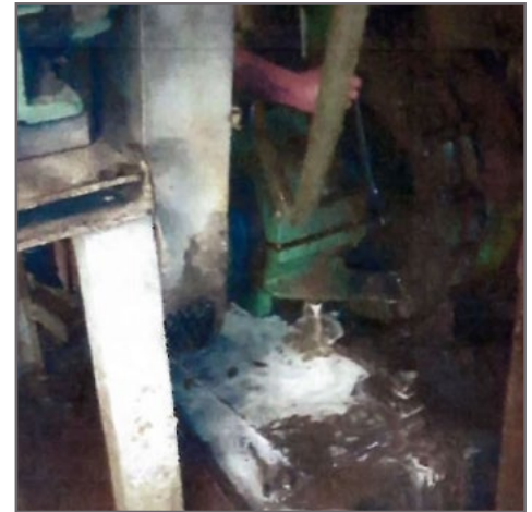
Flush water leakage all over the floor resulting hazardous operating conditions
