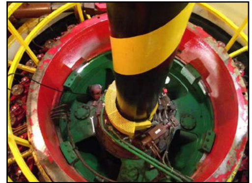
Voest Alpine Kaplan turbine with vertical axis
