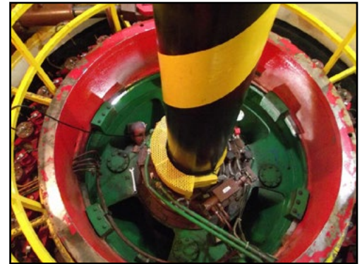
Voest Alpine Kaplan turbine with vertical axis
