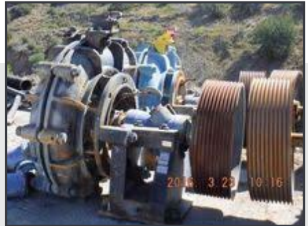
Warman Filter Feed Pump out in the open
