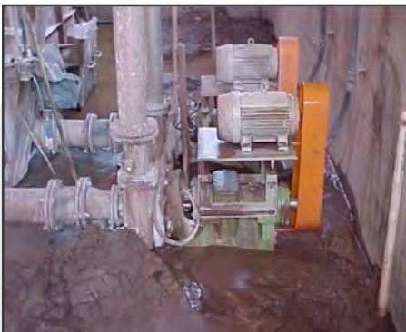
Product leakage, dirty environment before installation of SpiralTrac
