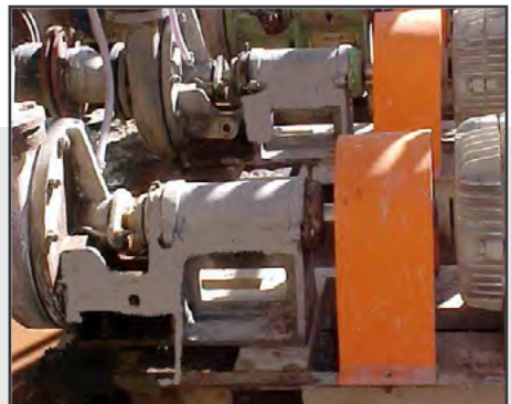
After installation of SpiralTrac the pump and surrounding areas remain clean and easily accessible
